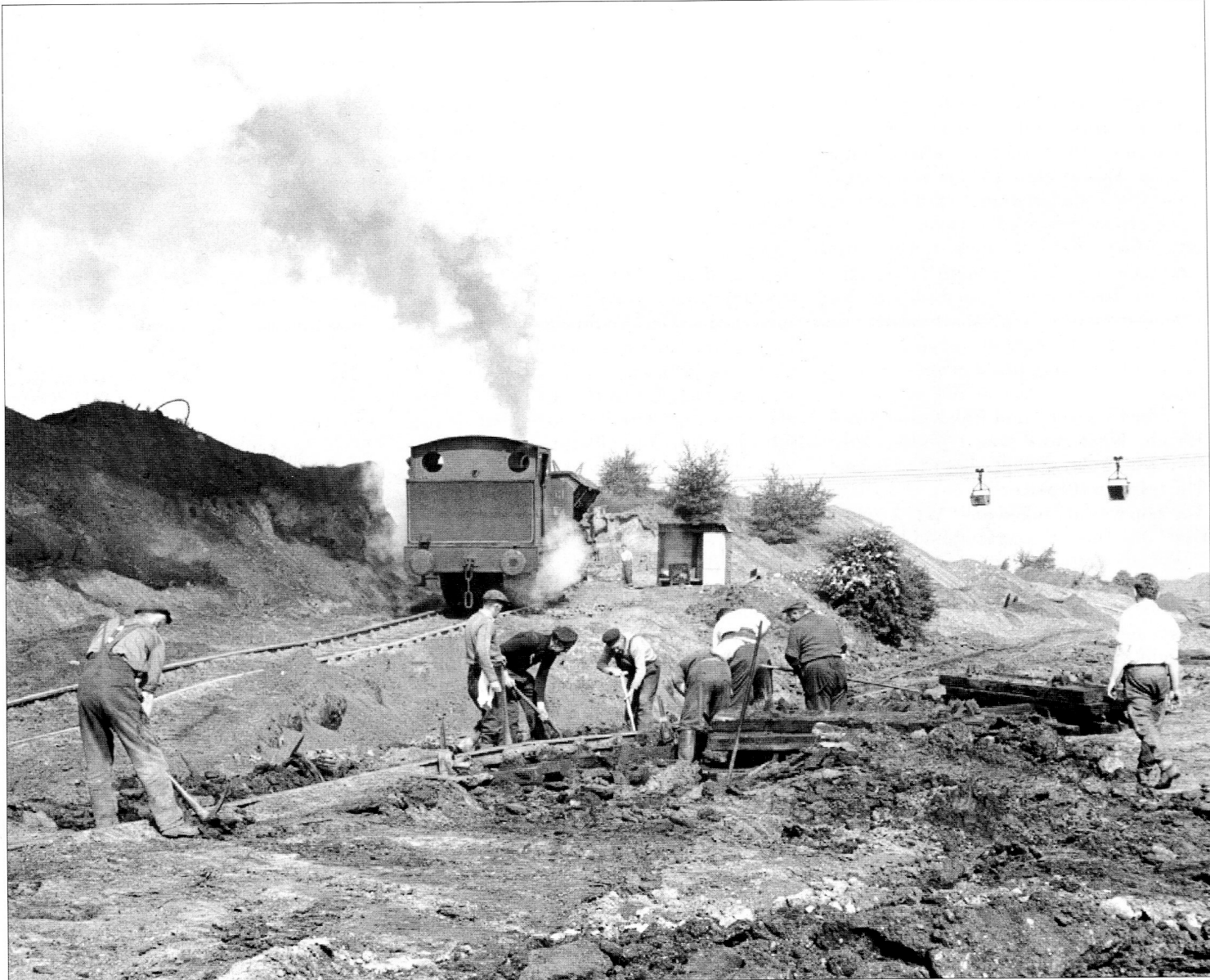
Elizabeth propels four side-tipping hoppers up to the spoil tip while platelayers are at work on the lower level track. The aerial ropeway can be seen in the distance. The date is 11 June 1969. PHOTOGRAPH: PETER STAMPER
